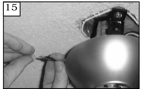
15 Make wire connections to power source using wire nuts provided. Make sure that no filaments are outside of the wirenut. After making the wire connections, the wires should be spread apart with the grounded conductor and the equipment-grounding conductor on one side of the outlet box and ungrounded conductor on the other side of the outlet box.
